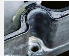
The edge of a CorroStall® aluminum alloy conduit box after the same salt spray test.
