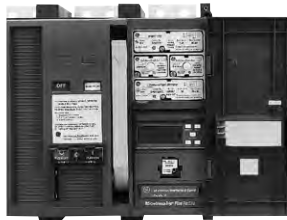
Breaker with limited access pushbutton cover assembly installed
