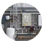
Panel Shops & Control Boards
