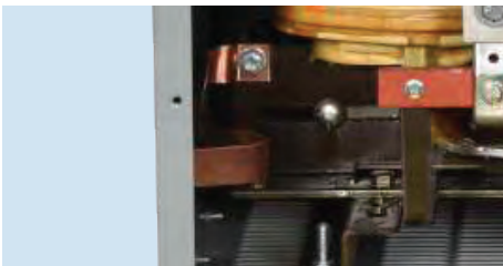
Factory installed main grounding lugs
