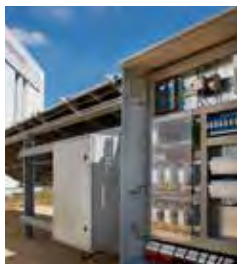
Pv Solar Test Lab
