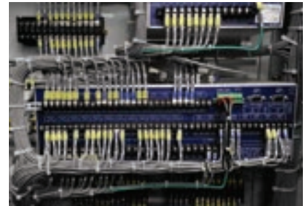
The installation of our customized wiring sets the industry standard for quality and efficiency
