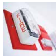
Fire & Safety Systems
