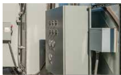
Rooftop Control Systems
