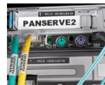
Network Infrastructure Labeling
