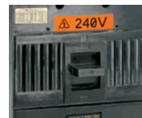
Electrical Hazard Labels
