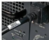
Electrical Infrastructure Labeling
