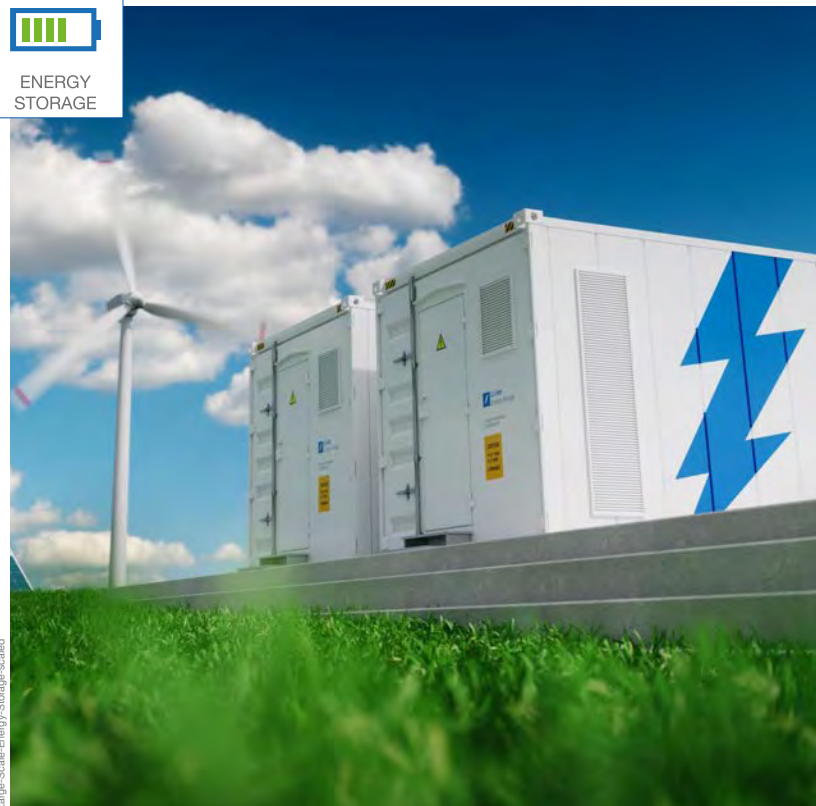
Large-Scale Energy Storage - outdoor
